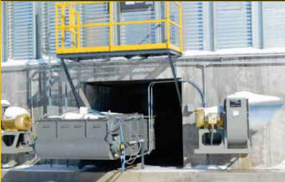
Hi Roller 60,000-bph reclaim enclosed belt conveyor at left and one of six Rolfes@Boone 50-hp centrifugal fans serving this 750,000-bushel Behlen tank.
