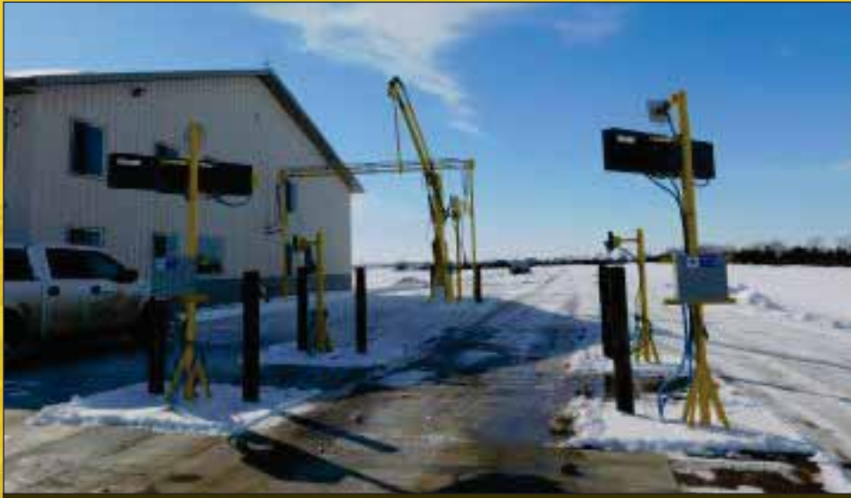
A pair of 120-foot Cardinal pitless scales under a oneWeigh scale automation system and a Gamet Apollo truck probe serve truckers entering and leaving the facility. Ground-level photos by Ed Zdrojewski.
