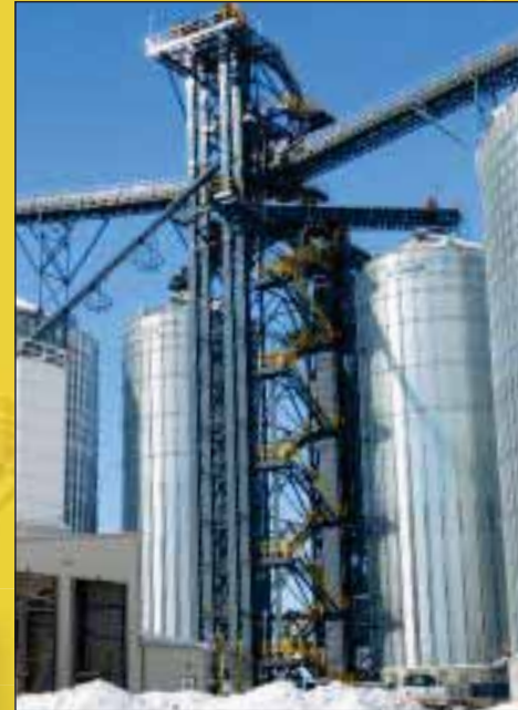
Warrior center tower with switchback stairs houses two Schlagel receiving and one shipping leg plus a Warrior screener and Schlagel distributor at the top. Twin enclosed receiving pits below left.
