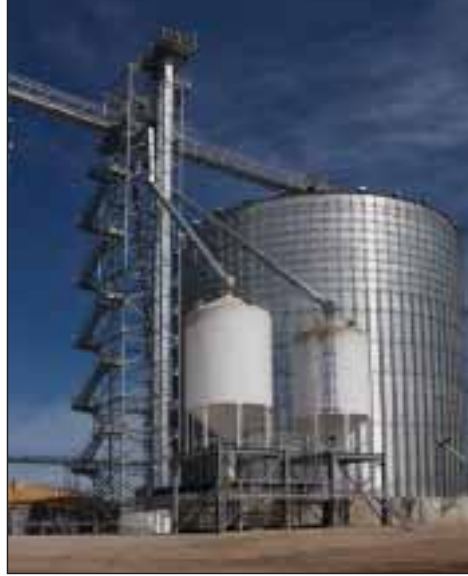
Ground view showing 15,000-bph Schlagel receiving leg in a 16-foot-x-16-foot LeMar tower, six-hole Schlagel rotary distributor, and two 4,000-bushel Meridian surge tanks.
